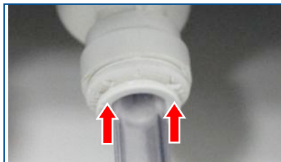
Fig. 87: Ring on drain valve
